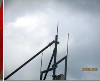
External photo(s) of the production unit(s) Lightning Protective System.JPG
