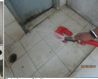
Photo of non-conformity NC 7.14 Water pressure flow of randomly checked fire hosepipe in 4th floor of main production building was not in acceptable condition.JPG
