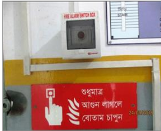
Photo of fire safety equipment Fire Alarm Call Point.JPG
