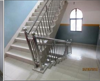
Photo of non-conformity NC 7.1 Hand rail was arranged at one side instead of both side of the stair.JPG
