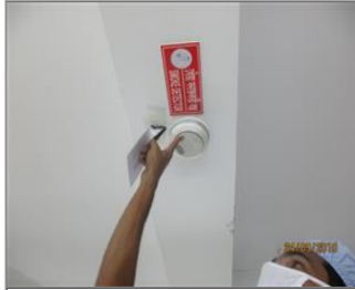
Photo of fire safety equipment Smoke Detector.JPG
