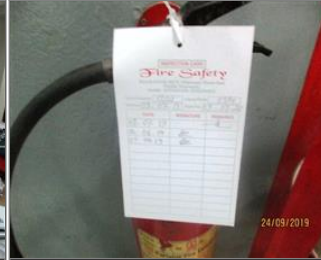
Photo of the inside of the main production hall Fire Equipment Inspection Card.JPG
