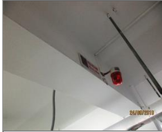
Photo of fire safety equipment Visual Fire Alarm System.JPG
