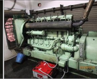
External photo(s) of the production unit(s) Generator Room.JPG
