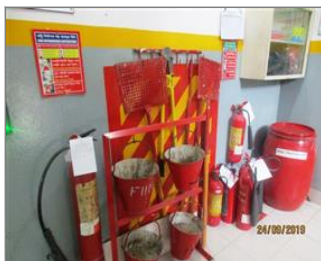
Photo of fire safety equipment Fire Fighting Equipment.JPG
