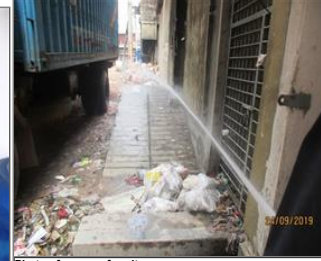
Photo of non-conformity NC 7.14 Water pressure flow of randomly checked fire hosepipe was not in acceptable condition on the ground floor of the main production building.JPG
