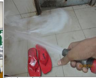
Photo of non-conformity NC 7.14 Water pressure flow of randomly checked fire hosepipe in 3rd floor of main production building was not in acceptable condition.JPG
