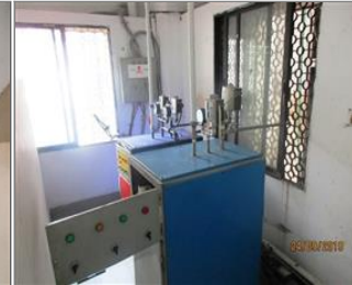
External photo(s) of the production unit(s) Electric Boiler.JPG
