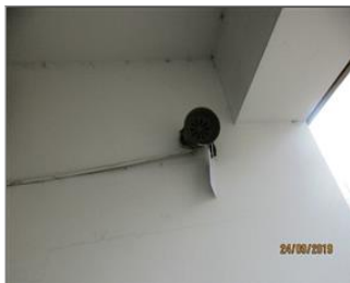
Photo of fire safety equipment Fire Alarm Sounder.JPG
