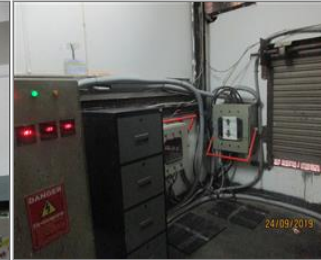
External photo(s) of the production unit(s) Substation Room.JPG
